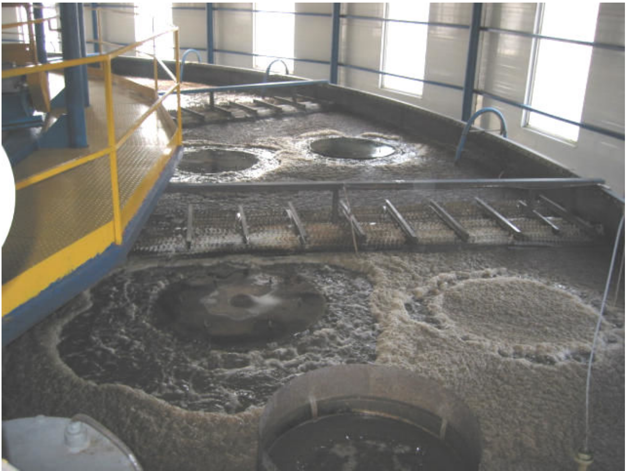
View of working aerators in sewage treatment in Paczków
